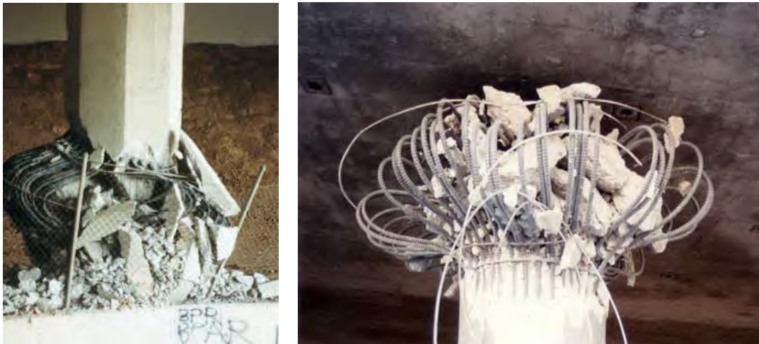
Figure 3.3 Failure due to strength degradation at plastic hinge regions of bridges damaged in the 1994 Northridge Earthquake (Caltrans 2006).
