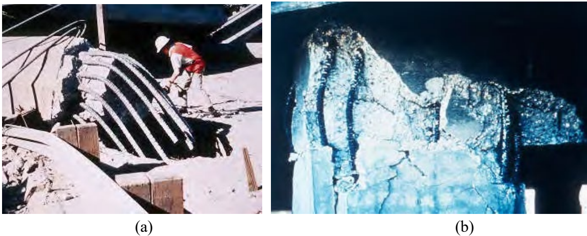
Figure 3.1 Pullout (a) and buckling (b) failure of bridge damaged in the 1971 San Fernando earthquake (Caltrans 2006).
